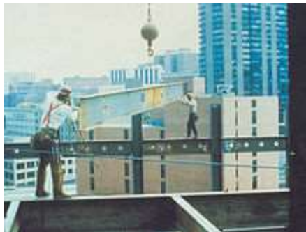
At-risk workers without appropriate safety equipment
